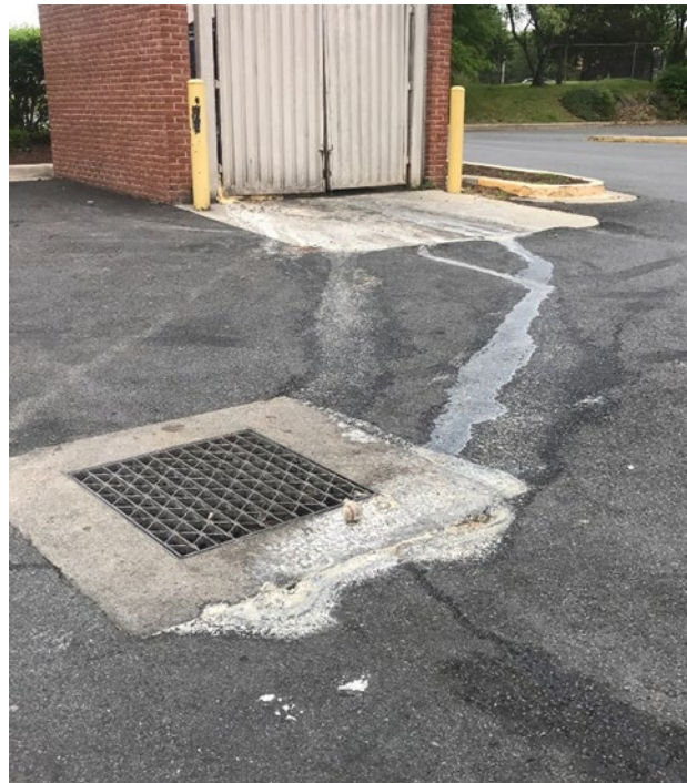
Illicit Discharge from commercial dumpster
