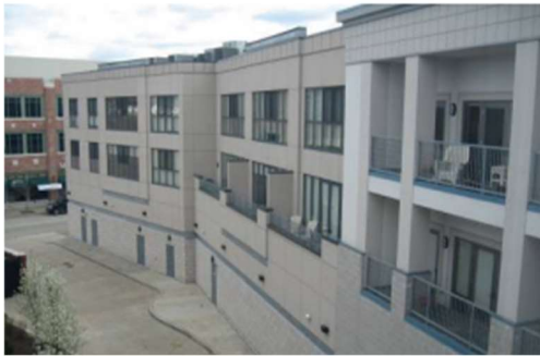
Inadequate parapet height exposes roof-mounted building/mechanical equipment.
