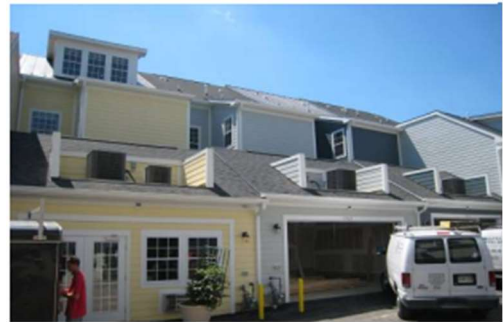
Exposed air conditioning unit in residential building can simply be treated with additional railing/ screen.
