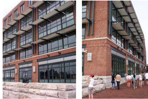
Sun shades can also serve to bounce natural light into the large open spaces within the building
