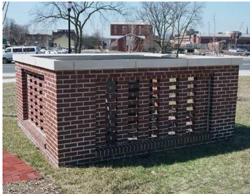
Vented brick enclosure wall for electric transformer
