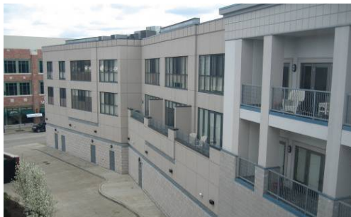
Inadequate parapet height exposes roof-mounted building/mechanical equipment
