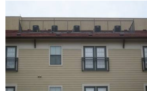
Rooftop utilities that are well located but insufficiently screened from view
