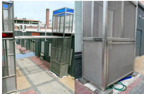
Vented stainless steel enclosure of gas and electric utilities and meters (Arts Alleyscape, Silver Spring, MD)
