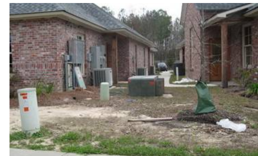
Electric and telephone transformers should be coordinated to minimize visual impacts on the corridor
