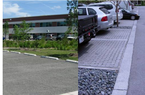
Permeable parking lot design using porous paving and permeable concrete to reduce stormwater runoff
