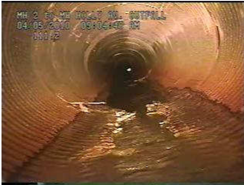
Photo 4 – 72” CMP – Corrosion of Pipe Bottom (typical)
