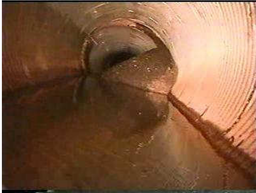
Photo 3 – 72” CMP – Breach 20’ Downstream of MH 2
