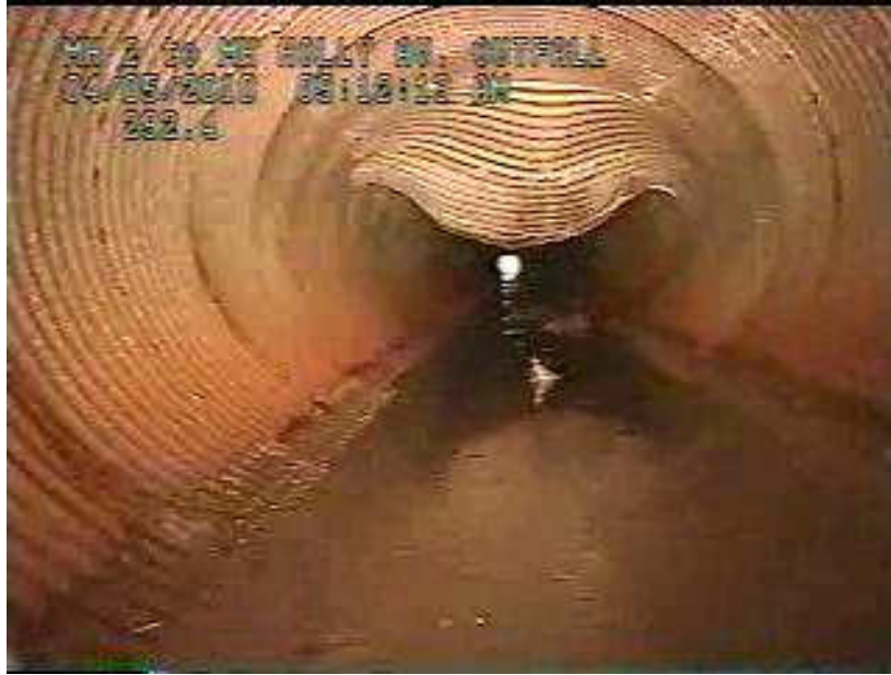
Photo 5 – 72” CMP – Pipe Breach 308’ Downstream of MH 2
