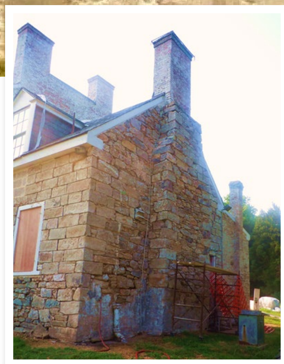
Pictured: West Wing restored. The inset depicts the West Wing with paint removed showing the cut and dressed stone construction and the fieldstone foundation.
