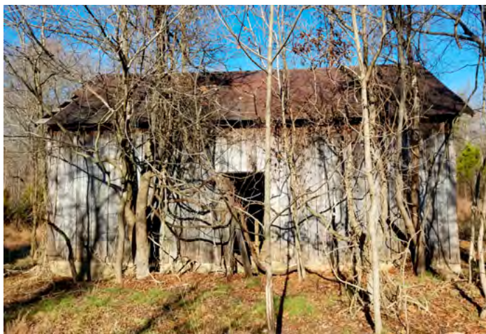
The outbuildings at the Epp Farmstead were typical of those throughout Southern Maryland and did not reflect characteristics commonly associated with German architecture.
