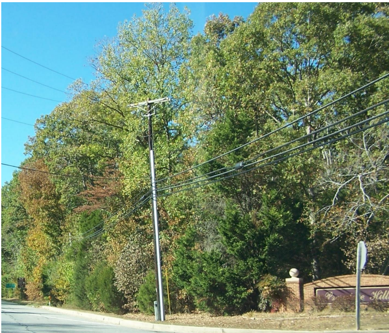
Figure 11: Utility Pole Requiring Make-Ready
