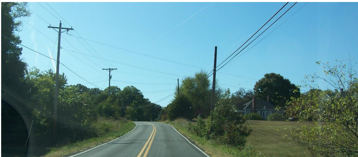
Figure 13: Low-Make-Ready Pole Line in Unserved Area with Communications on a Separate Pole
