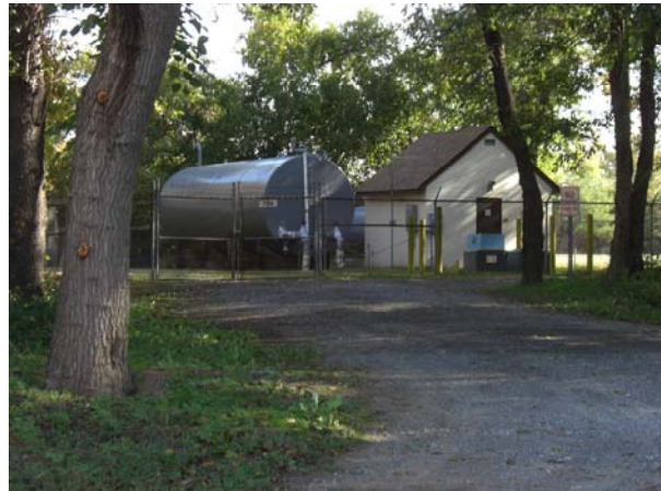
Fig. 2-13 – The existing County-operated community water supply facility adjacent to Benedict Avenue
