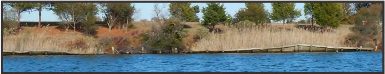
Figure 6-4. Failing bulkhead, Site 55, recommend replace with Type 4 sill.
