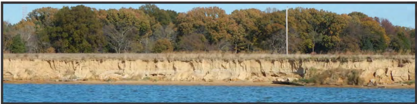
Figure 6-5. Eroding agricultural upland, Site 61, designated P-2 and recommend Type 5 sill.
