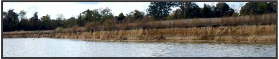
Figure 5-4. Reach 1-B – Site 23, recommend a Type 3 sill; a designated P-1 site, eroding upland, farm field with no wood buffer.
