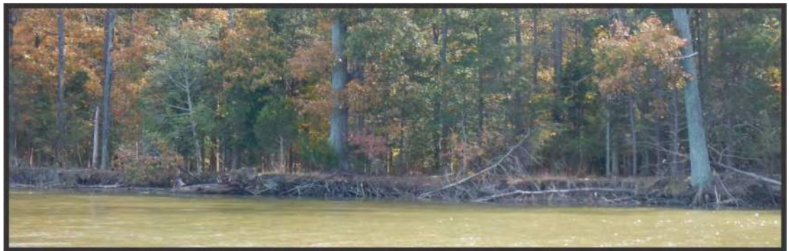
Figure 5-2. Reach 1-A – Eroding wooded upland bank, Site 2, Type 1 sill recommended.
