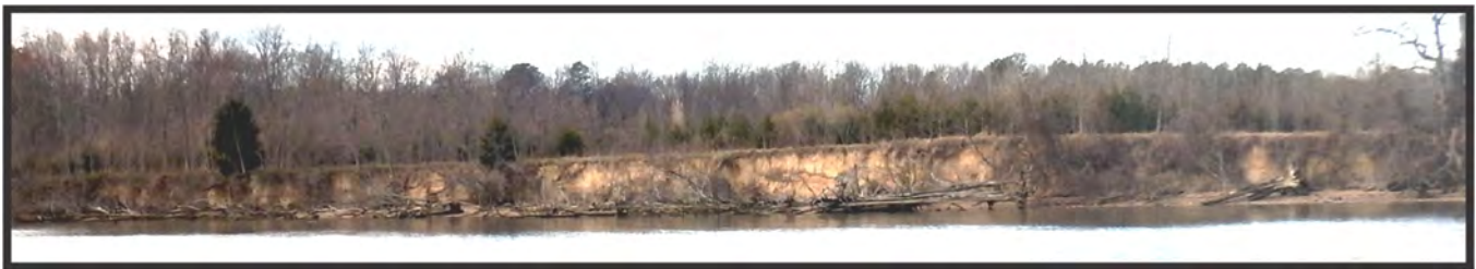
Figure 8-2. Eroding low agricultural upland bank, Site 96, ranked as a P-2, recommend Type 5 sill.
