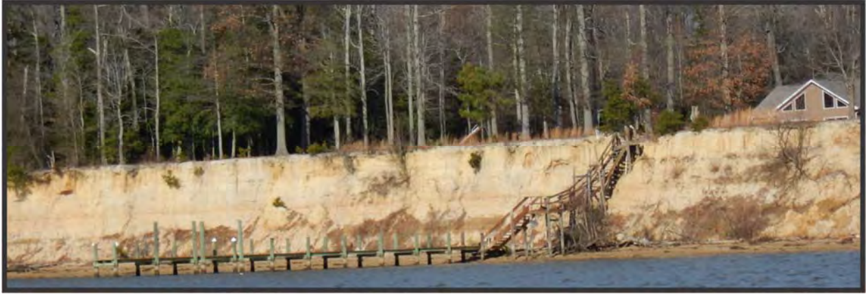
Figure 9-2. Vertically exposed eroding upland bank on residential property along Reach VA, Site 115, recommend Type 5 sill.
