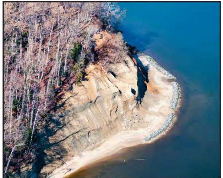
Figure 4-4. Brill system soon after construction at Westmoreland State Park in Virginia. These large structures are more continuous than breakwaters, but they are farther offshore than a sill. Eventually, the backshore will begin to vegetate.
