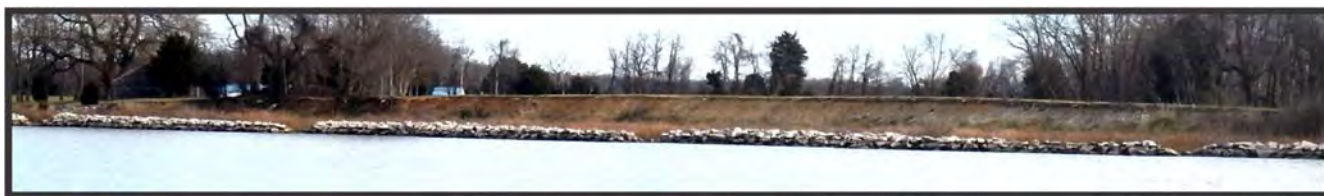
Figure 8-3. Along Nanjemoy Creek, a low upland bank protected by a gapped sill system exists, but the bank was not graded. This type of system is comparable to a Type 4 sill system.
