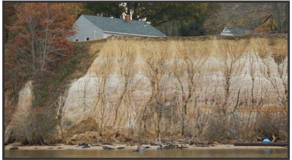
Figure 10-4. Eroding high bank with upland runoff problems as evidenced by gullies running down the bank. Site 144, Type 5 sill, bank grading recommended. Nearshore is deep and may restrict options to shoreline defense, like a revetment.
